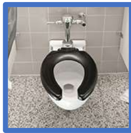
Flushometer Valve Toilets
