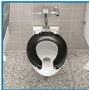
Flushometer Valve Toilets
