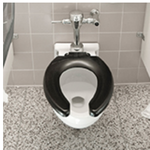
Flushometer Valve Toilets
