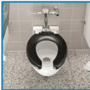
Flushometer Valve Toilets
